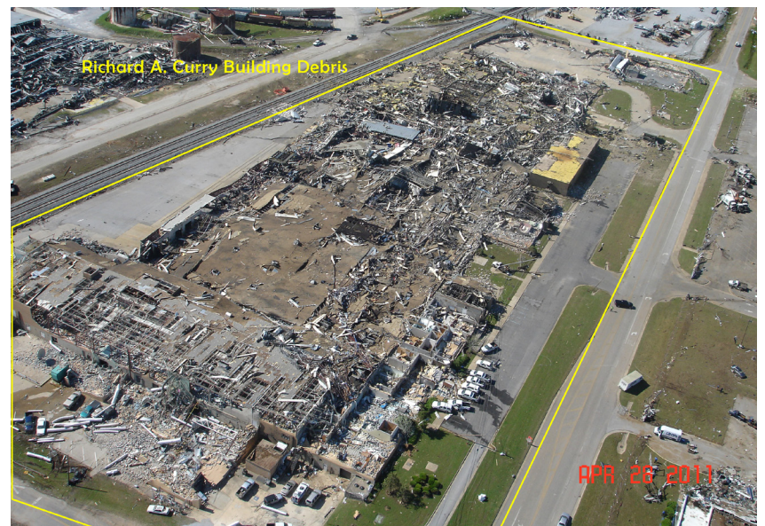
Aerial photograph of what's left of the Richard A. Curry facility on April 28, 2011.
